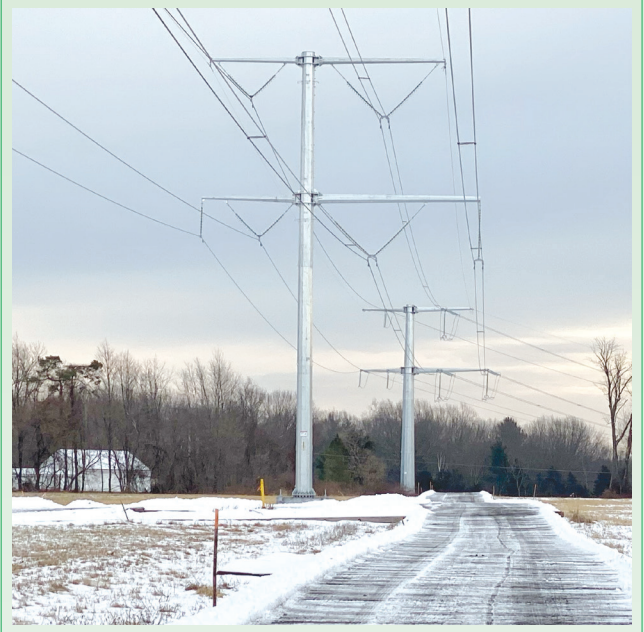
New NYES monopoles are delivering more clean energy.
